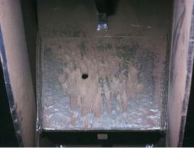
Wear in the ventilator
